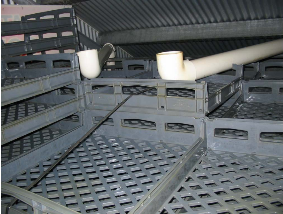
Figure 12.1: Tray aerator made from bread crates at Pleasant Point
